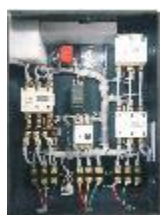
Interior View of MU-G30W FASD
